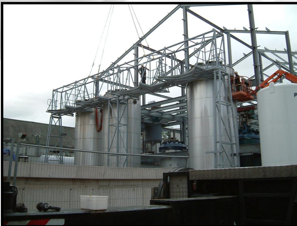
Left: One of slinger/banksman guiding a vessel into position so as not to damage the aluminium lagging.
