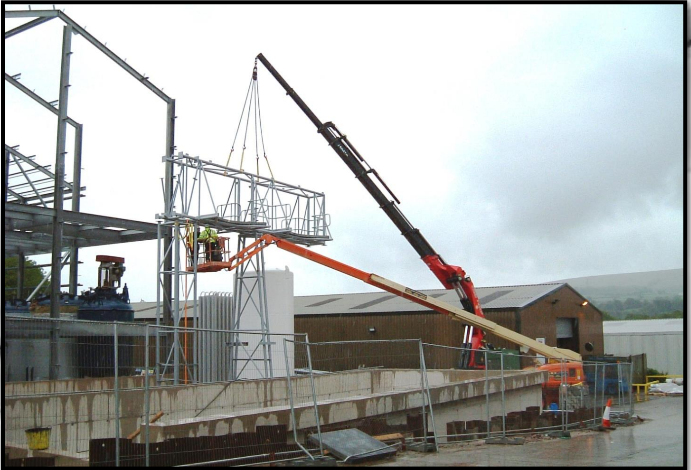
Above: Installing the newly engineered walkway onto the legs. The weather has decided to take a turn for the worse.....again!
